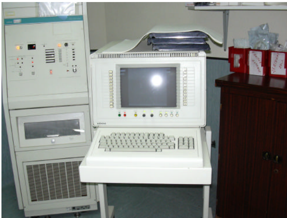
Figura 27: Digital Operator’s Terminal (DOT) with Digitrac
