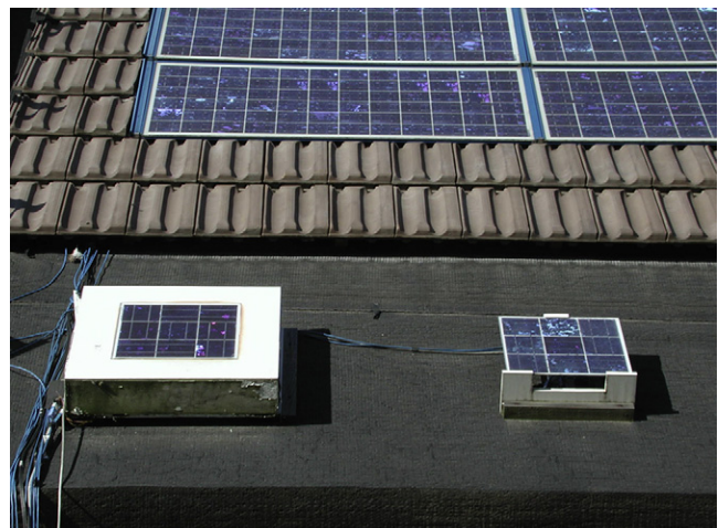
Fig. 4. Different BIPV conditions: integrated roof (top), ICT reference device (on the left) and ventilated reference device (on the right) [7].
