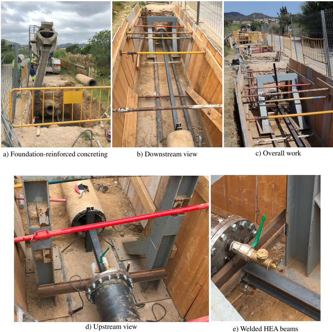
Figure 5.7: Detailed setup for fixing the blind flanges to withstand 25 bar in a DN 400 mm pipe: foundation-reinforced concreting (a), detail of the downstream view (b), general view of the work (c), detail of the upstream view (d), and detail view of the welded HEA beams (e).
