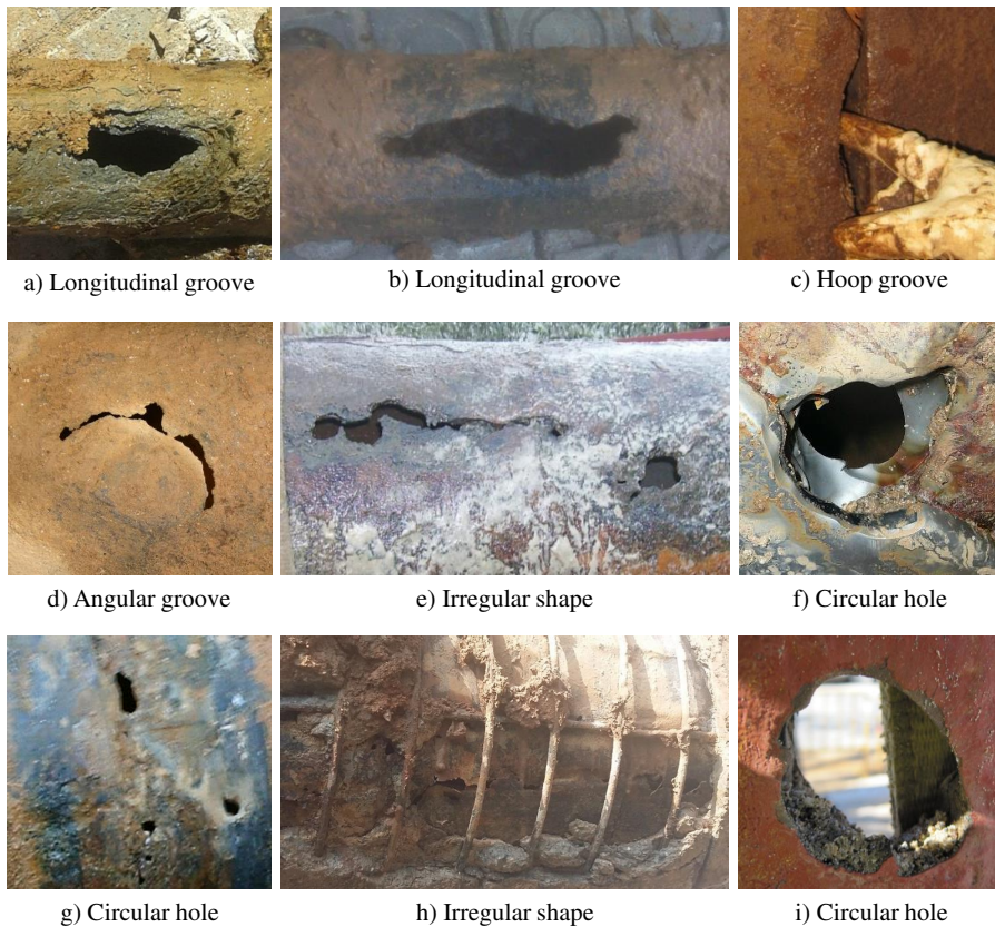
Figure 2.19: Holes typology reported in real host pipes. Circular-like holes (f-g, i), longitudinal grooves (a-b), hoop grooves (c), angular grooves (d) and completely irregular shapes (e, h).
