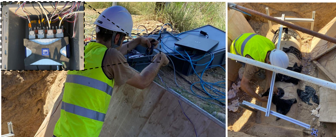
Figure 5.11: Installation of the middle section liner's strain gauges under challenging field conditions (July, Barcelona).
