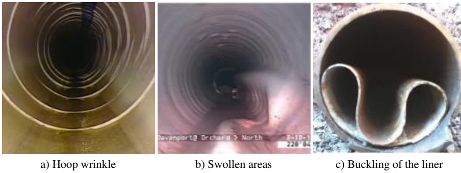
Figure 3.2: Defects caused by difficulties in the installation of the liner: hoop wrinkles (a), swollen areas [94] (b), and the buckling of the liner [94] (c).
