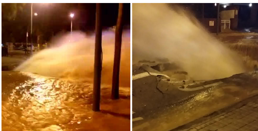
Figure 1.1: Example of real pressure pipe failure causing important damage to the road and third parties.
