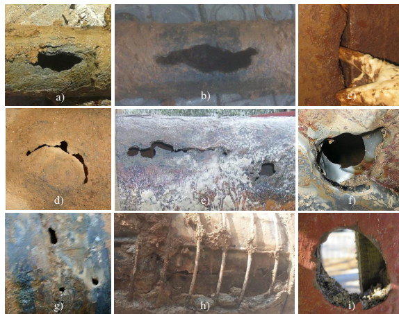
Figure 1: Examples of holes detected in damaged pipes.
