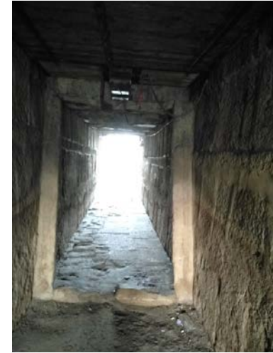
Fig. 154. Embedded stone edges supporter for keeping the wooden boards' frames inside the water corridors, Khaju Bridge. taken by the author
