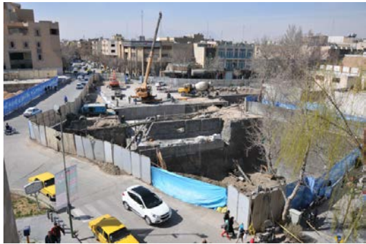
Fig. 306. Maidan-e-Darvazeh Dolat, Construction of the metro entrance at the place of the city's first gas station, February 2016. Source: author
