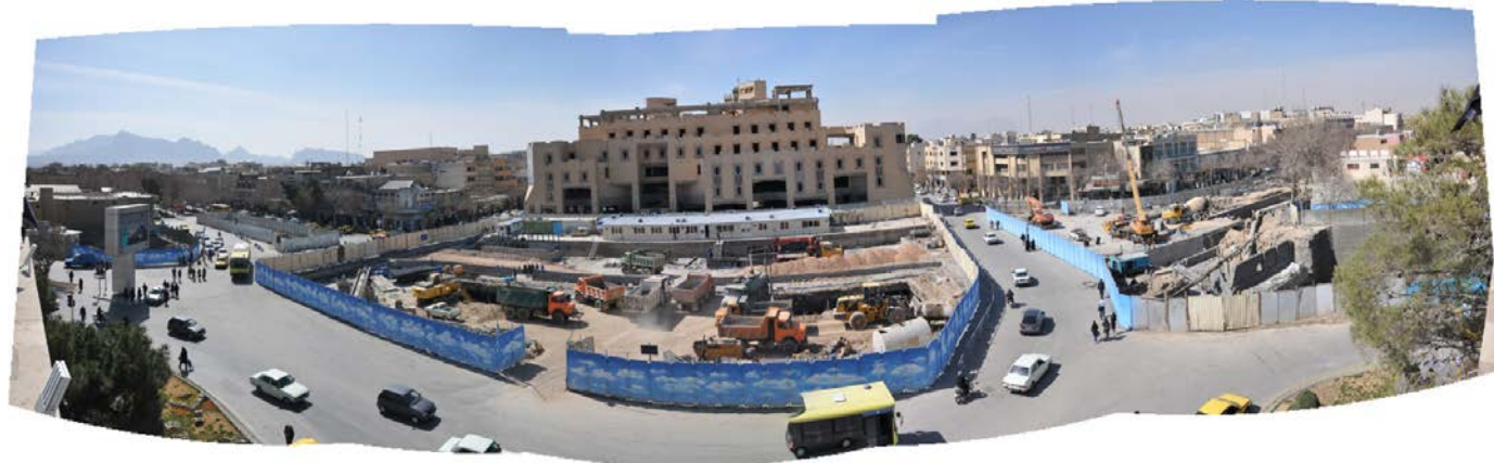
Fig. 313. View from the top of city hall to Maidan-e-Emam Hossein, and Jahan Nama center, February 2016. Source: author
