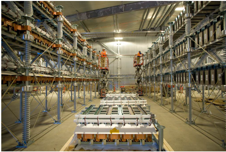
Fig. 1.5: Converter hall for Trans Bay link. Photo courtesy of NextEra Energy, Inc.
