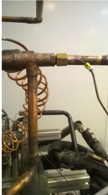
Figure 2.30. Immersion thermocouple at the exit of the IMS subcooler.
