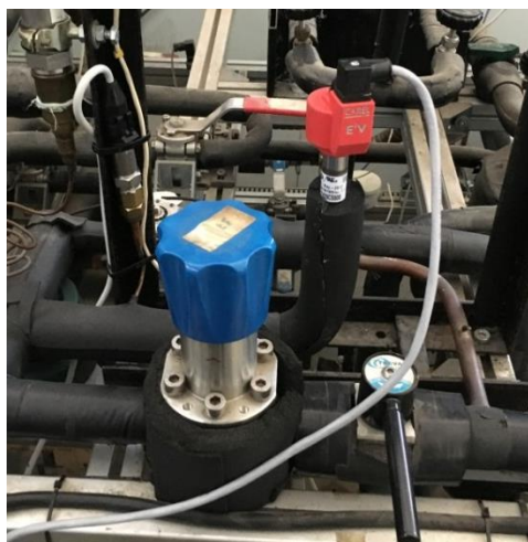
Figure 2.5. Previous back-pressure valve (blue) and new electronic back-pressure valve (red).
