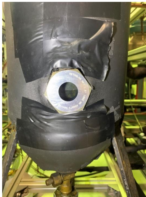
Figure 2.9. Liquid vessel sight glass with liquid level.
