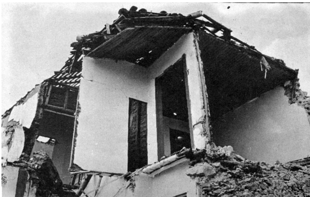
Figure 2.23. Image of the destruction generated by the 1969 Horseshoe earthquake in the Lisbon region. From CERU, (2015).
