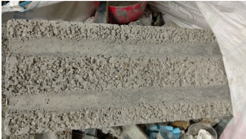
Figure 38. Voids in concrete
