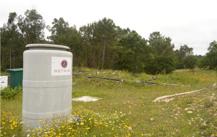
Figure 4.2. Overview of the hydrolytic upflow sludge blanket (HUSB) reactor and the full-scale constructed wetland system for winery wastewater treatment located in Galicia (Spain).
