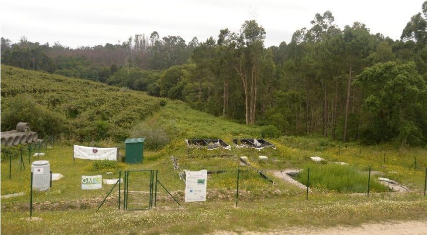
Figure 4.1. Overview of the full-scale constructed wetland system for winery wastewater treatment located in Galicia (Spain).
