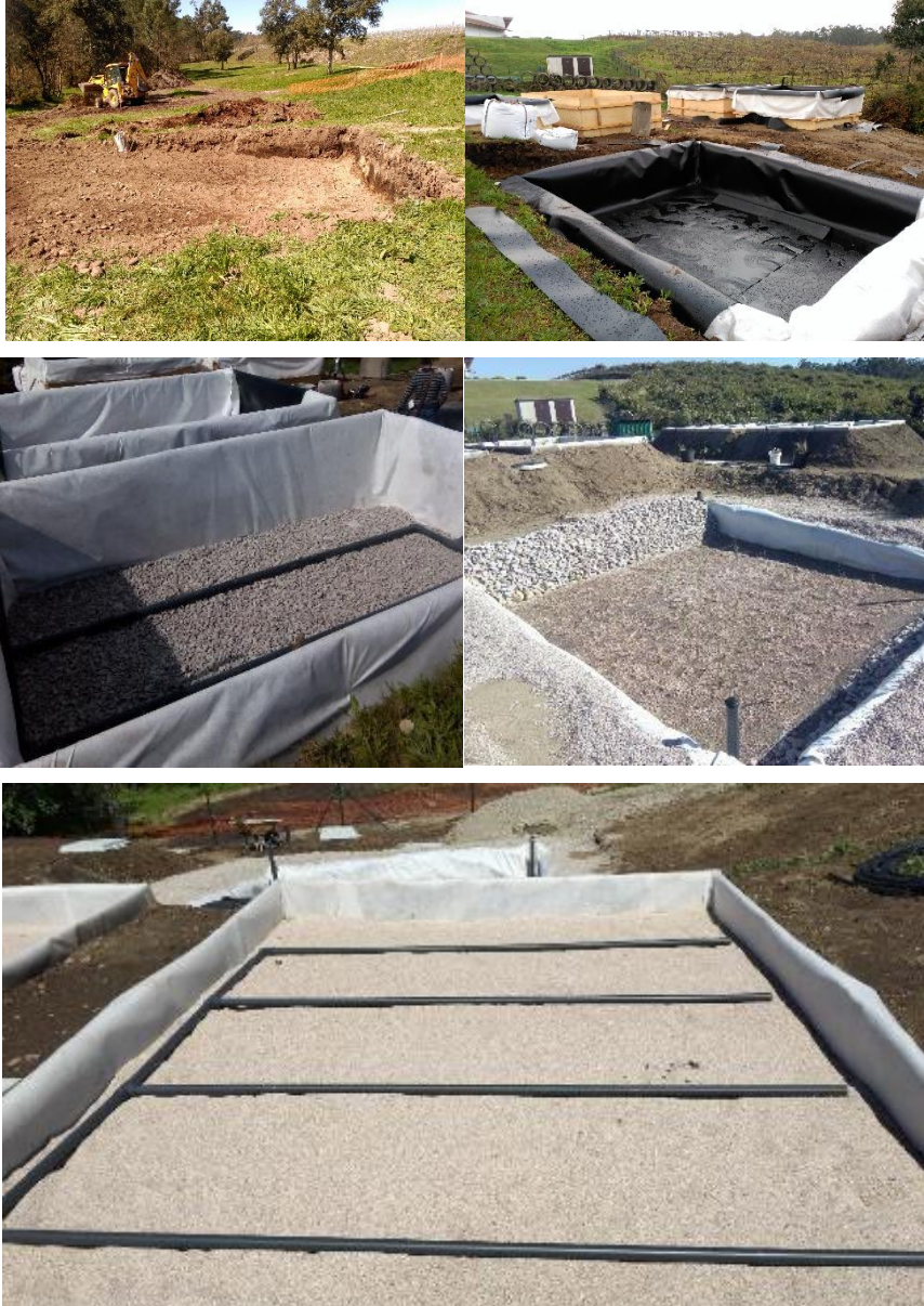
Figure 4.6. Construction phases of the full-scale constructed wetland system. Earthmoving (top left), impermeabilization (top right), drainage pipes installation (middle left), filling of filter media (middle right), feeding pipes installation in the vertical subsurface flow constructed wetland (bottom).
