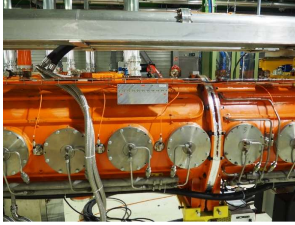
Fig. 6.4. CERN SPS travelling wave cavity in BAF3 test-stand during the Long Shutdown 2, before installation in tunnel.
