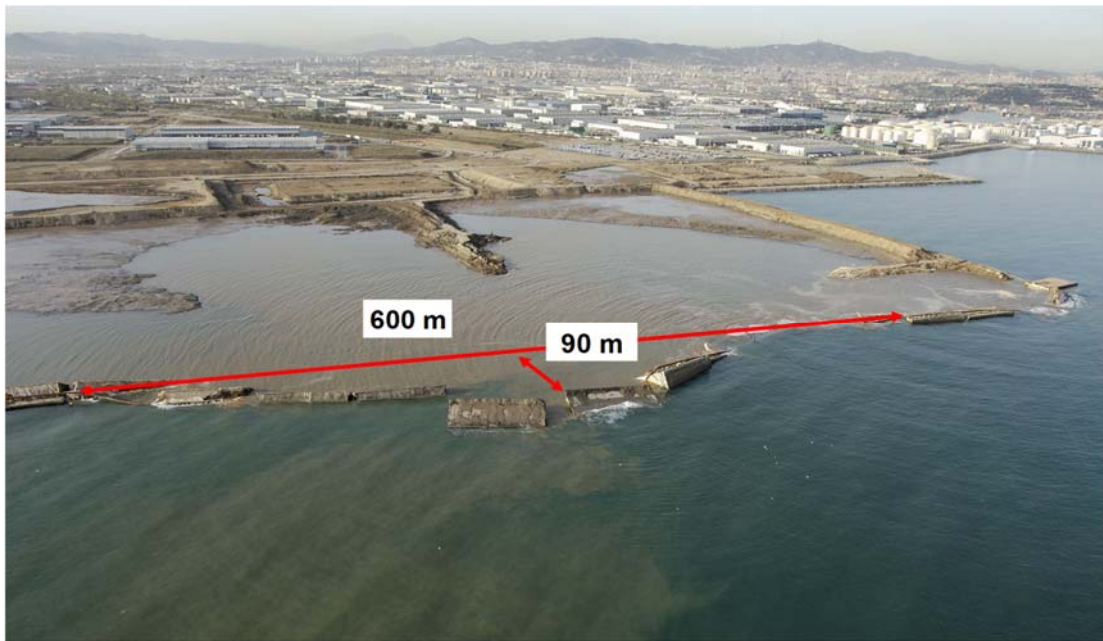
Figure 2.18. Aerial photo of Phase 1 of the failure (Courtesy of Barcelona Port Authority).
