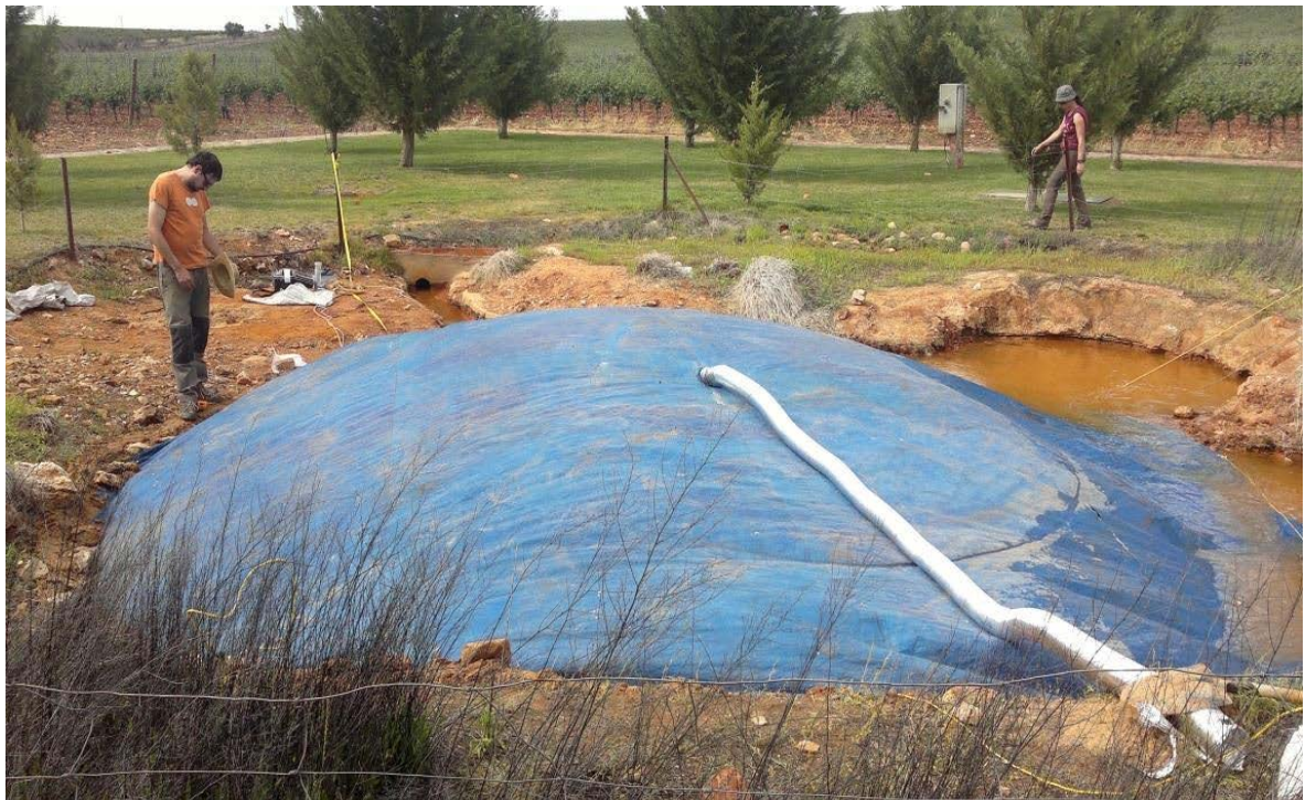
Figure 23. The SAP system installed and working at Cañada Real site. Note the pipe connected to the centre of the blanket to determine gas flux.
