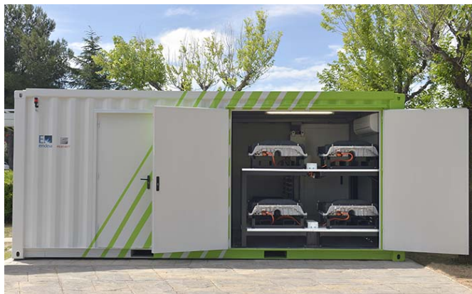
Figure 3.4: SUNBATT container located at technical centre of SEAT (Martorell - Barcelona)
