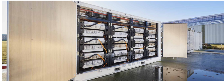
Figure 3.10: Renault Second Life Batteries project in Belgium
