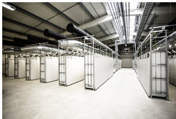
Figure 3.9: Second Life Batteries project in Elverlingsen in Germany
