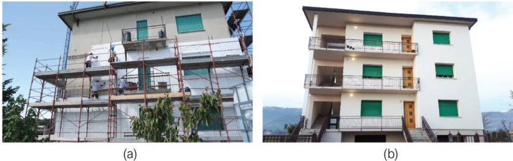
Figure 1.9. Example of the retrofitted building with the ECOSISM Seismic Coat before (a) and after (b) the restoration [12].
