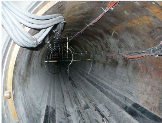
Figure 4.12: convergence sensors installed on the insert.
