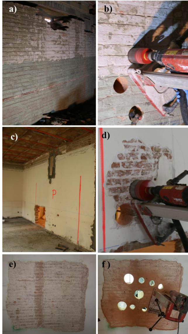
Figure III.8 a) Façade wall investigated in “Fabra i Coats” factory and b) in-situ core drilling for campaign “MB”, c) inner wall of the analysed building in Rambla Catalunya street and d) in-situ core drilling for campaign “MC”, e) inner wall of the building in Ciutat Vella and f) in-situ core drilling for campaign “MD”.
