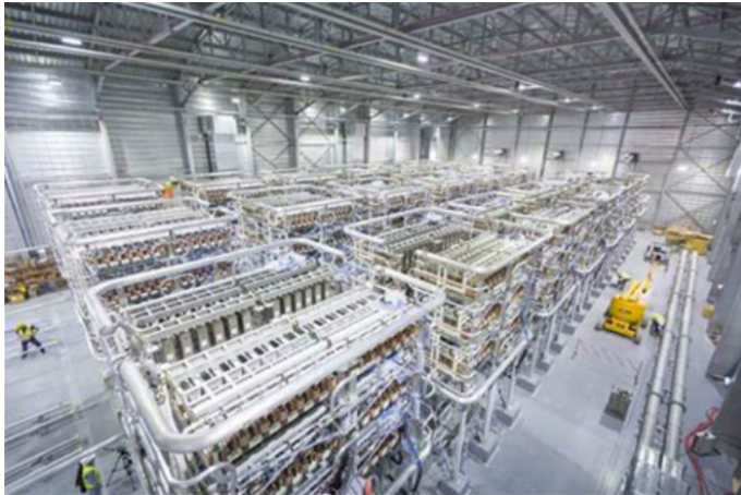
Fig. 1.9: INELFE project – MMC (Courtesy of Siemens)
