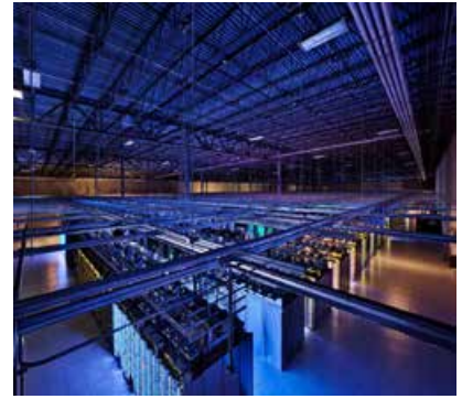
FIG. 30 Google, Council Bluffs data Centre, Iowa, EE.UU.
