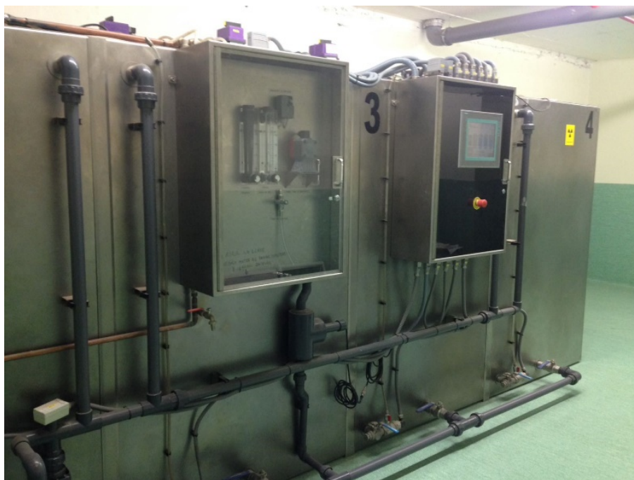
Figure 1.5: Holding tanks for urine storing from confined patients' treated with ^{131}\text{I} located in the basement from one BMA hospital.
