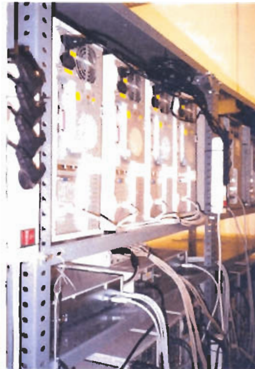
Figure A.3: Back of the switches and connections
