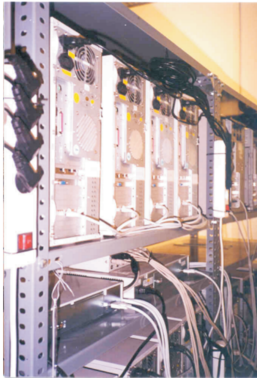
Figure A.3: Back of the switches and connections
