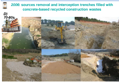
D) Sequential images of pollution sources removal and construction of current trenches. E) Schematic representation of proposed hydrogeological performance of the interception trenches. Rainwater leachates contaminants retained in the unsaturated zone and infiltrates to the trenches. The water table level of trenches represents the minimum level.
