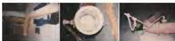
FIG. 6. Discharge piping, circular valve and valve actuator.
