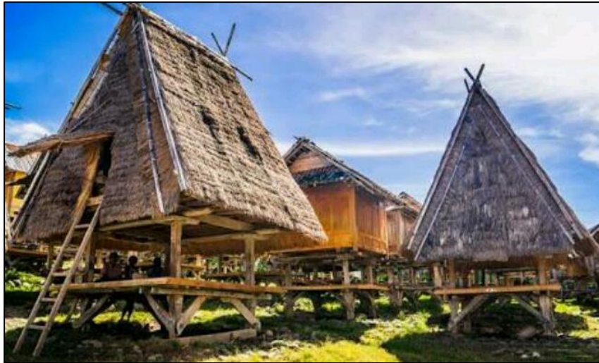
Fig.163: Sumbawa houses (Indonesia) in case of necessity holes can be easily obtained piercing the walls made of bundle of reed ( http://muhamadyasid.blogspot.com ).
