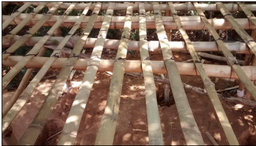
Fig.114: Two details of the Sri Ma (Auroville, India) house base plane and its connection system ( www.auroville.org )
