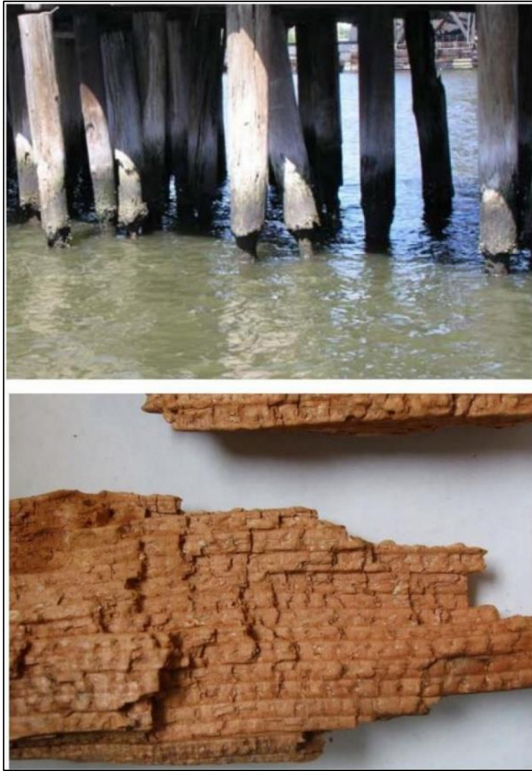
Fig.64. Upper: in order to rot, wood needs oxygen and water. Therefore, the rot will occur on the surface of the water (Fraaij 2007). Lower: wood rot (Fraaij 2007).
