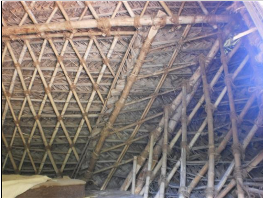
Fig.142: Roof detail of a Sri Ma house base plane (Auroville, India) showing the overhead framing. The elements are tied together using ropes made of natural fibres ( www.auroville.org ).
