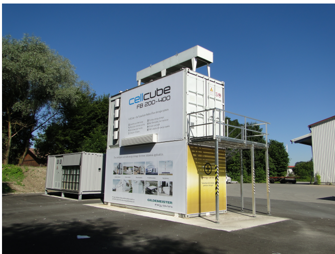
Figure 1.2: The vanadium redox flow battery installed in the SmartPower-Flow project.
