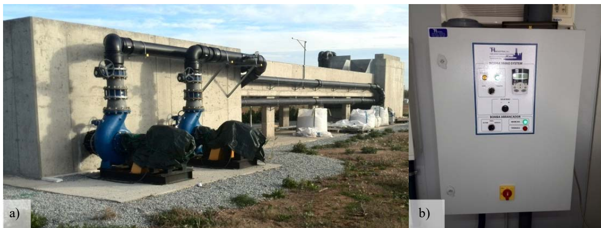
Figure 2.3- Pumping system (a) picture and (b) VFD.
