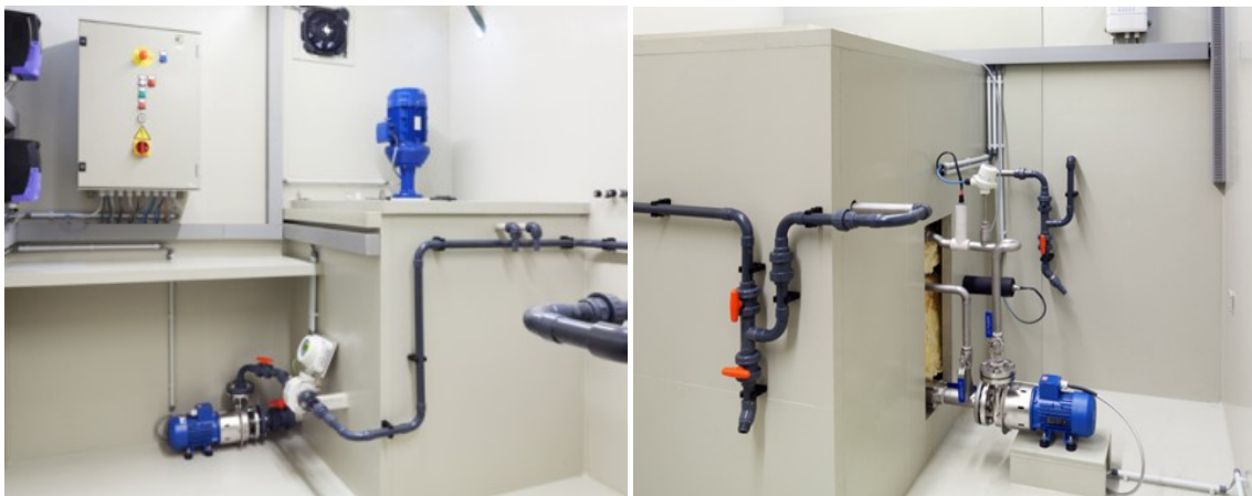
Figure 2.6. General view of the anaerobic digestion (AD) pilot unit.
