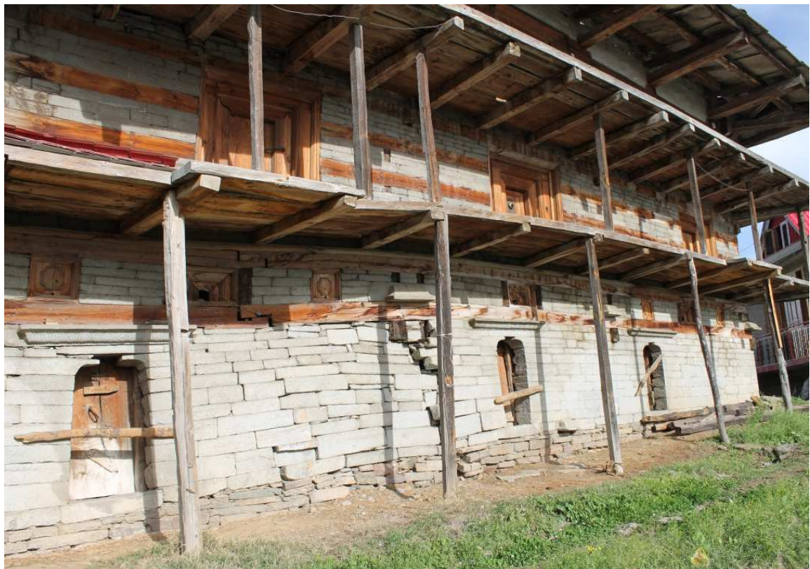
Figure 4.5 Cracks in village homes due to blasting for tunnels inside the mountains. Area of Sawra Kuddu dam, April 2015. Photo: Daniela Del Bene
