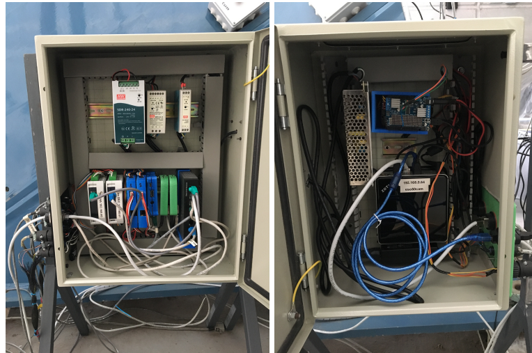
Figure 5.3.3: The new control box and electronics of the 50cm telescope. The TCS and associated subsystems are embedded in the left-hand box, while imaging-related equipment has been installed in the right-hand box
