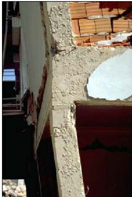
Picture 12: Damage to beam-column joint, large rotations at the end of the columns. Building in Adapazari, Turkey [PEER, 2000].
