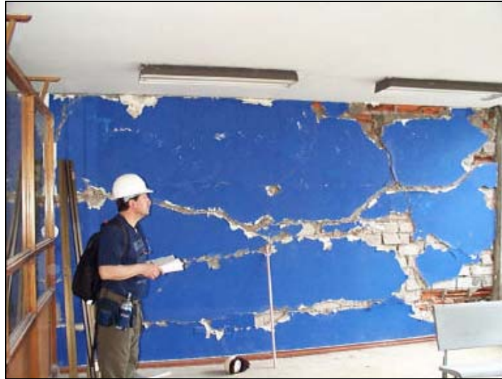
Picture 6: Damage in masonry wall (3 rd floor), building in Pereira, Colombia [Pujol et. al, 1999].
