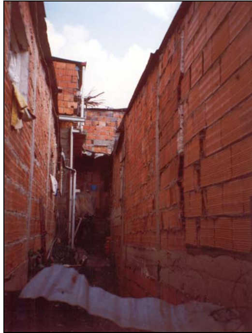
Picture 14: Alley in the Cristo Rey Sector showing four houses, the low quality of workmanship and materials in the walls and the absence of collar beams is observed.
