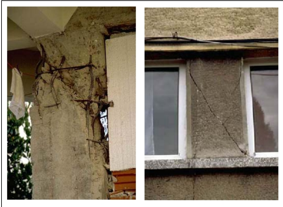
Picture 11: Damage in columns. Left: Shear and axial failure due to excessive stirrup spacing. Right: shear failure in captive column. Building in Adapazari, Turkey [PEER, 2000].
