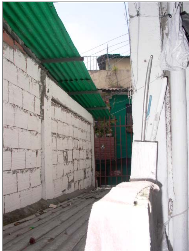
Picture 5: Metallic sheathing roofing. Poor bonding to frame and walls.
