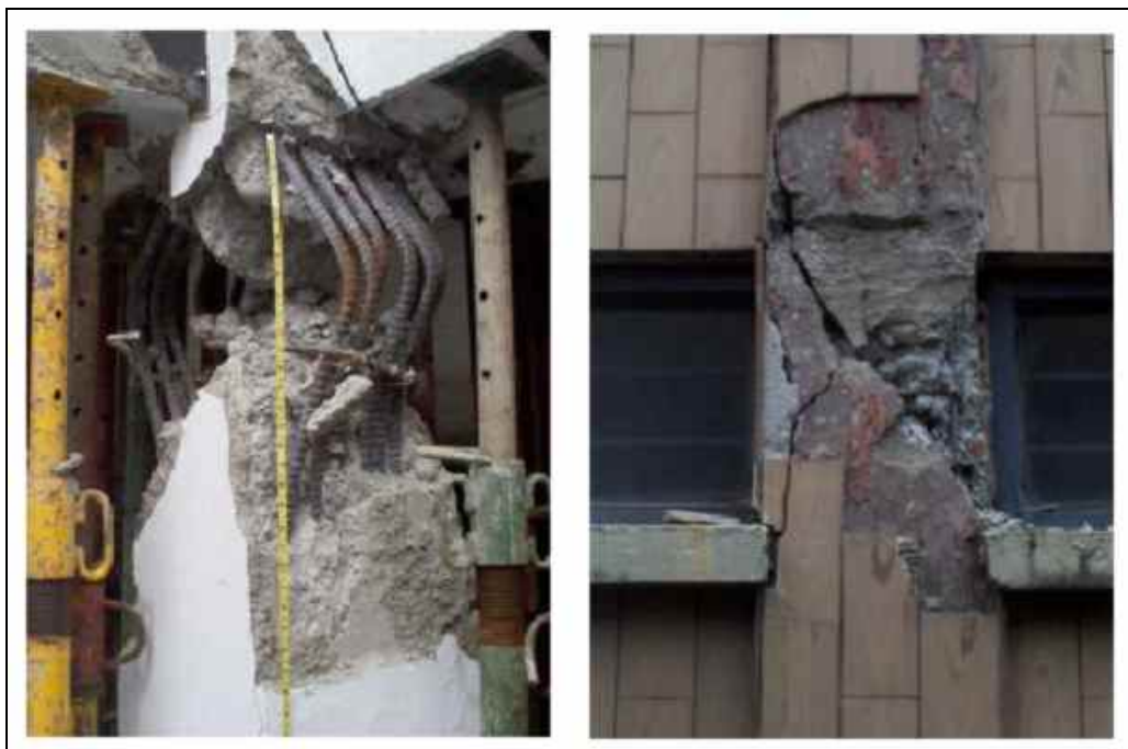
Picture 8: Damage in columns. Left: buckling of longitudinal reinforcement due to the lack of adequate transverse reinforcement. Right: Short-column effect. Both buildings in Armenia, Colombia. After [Pujol et. al, 1999].
