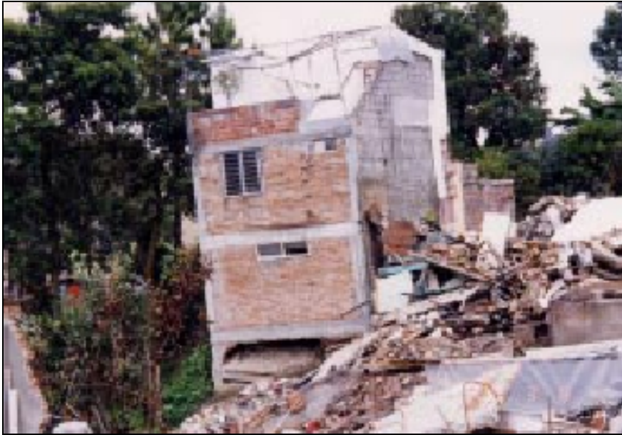
Picture 9: Damage in building due to steeped soft soil. Building in Armenia, Colombia. [Yoshimura et. al, 1999].
