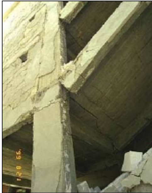
Picture 10: Beam damage, longitudinal reinforcement slippage. Building in Adapazari, Turkey [PEER, 2000].
