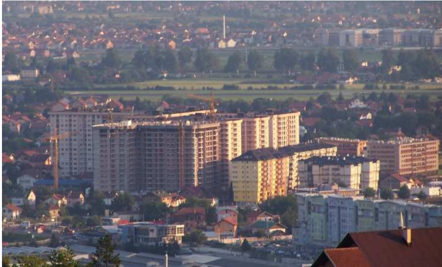
Figure 11. Construction of multi-family housing by Tibra Pacific in Stup (Ilidža). Source: sarajcity.com
