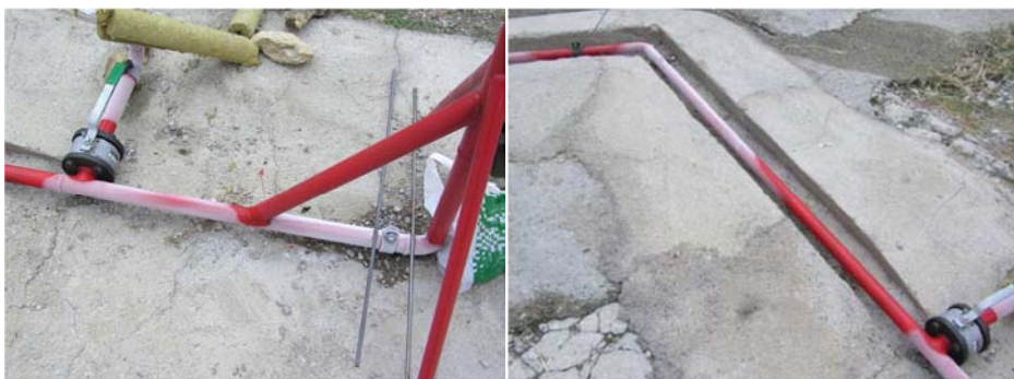
Figure 2.18. View of the frozen pipe due to the existence of two-phase flow.
