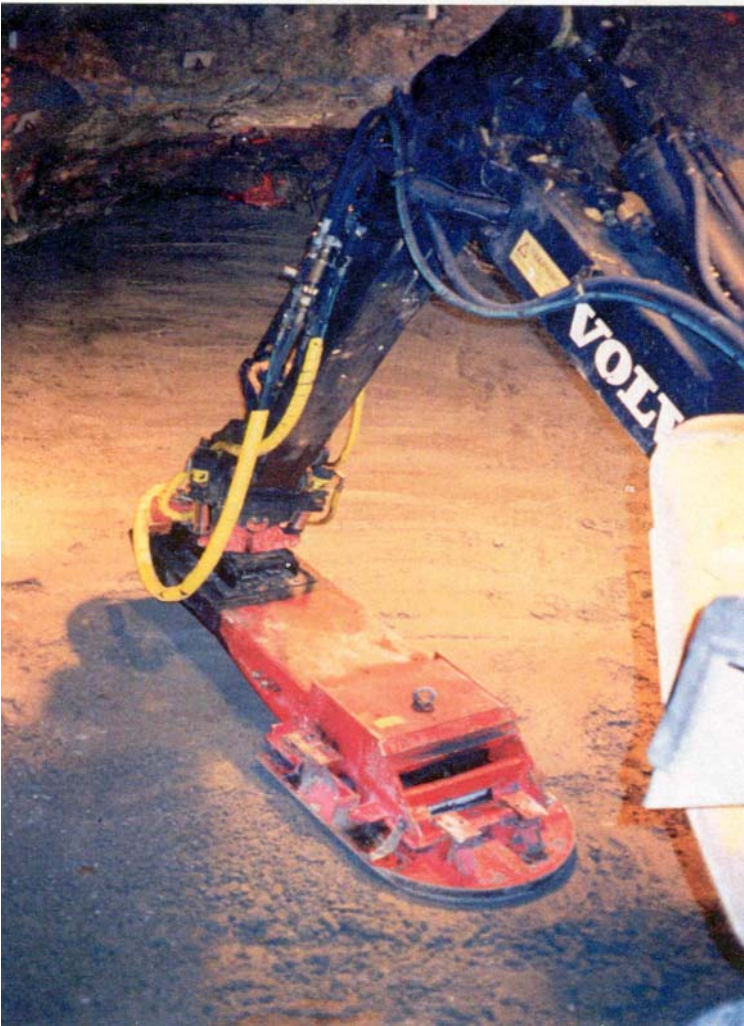
Figure 2.9: Designed facility to compact the backfill far away from the roof (Gunnarsson et al. 2001).
