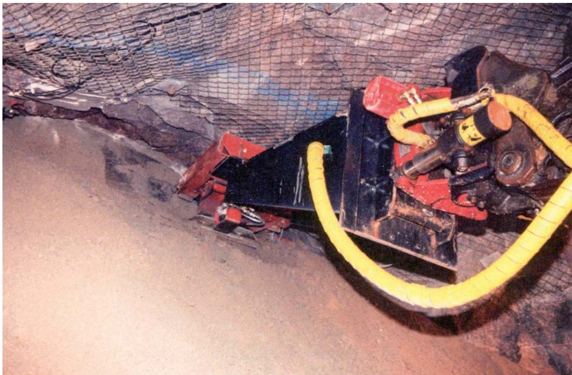
Figure 2.8: Designed facility to compact the backfill close to the roof (Gunnarsson et al. 2001).
