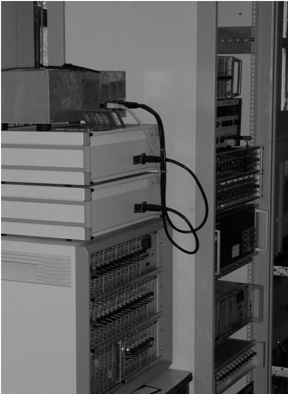
Figure D.4 64-channel amplifiers
