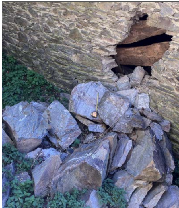
Figure 2: Deposit of the Pont de Gulleri (PdG) rockfall event, stopped against a stone home wall.
