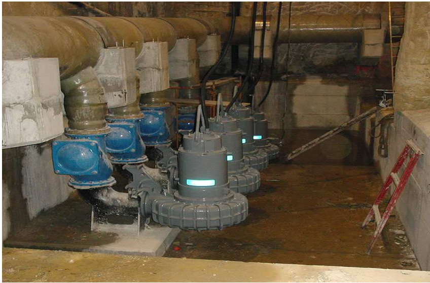
Figure 2.6: Typical pumping station for reservoir. Taken from [CLA05].
