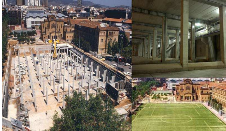
Figure 3.6: Retention tank located at Escola Industrial de Barcelona.
