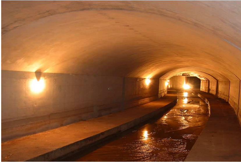
Figure 2.2: Big diameter sewer. Taken from [CLA05].
