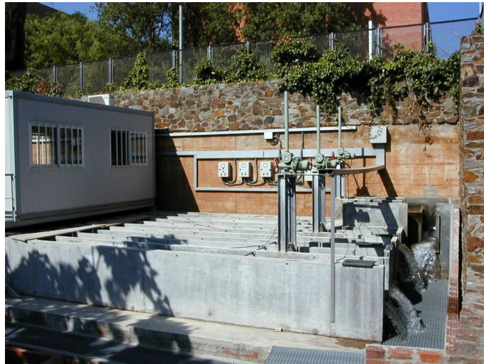
Figure 3.2: Lateral view of the Canal PAC-UPC in operation
