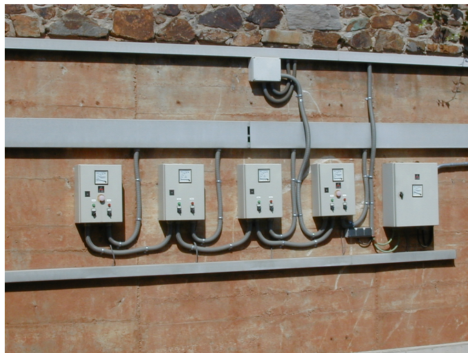
(b) Control boxes
