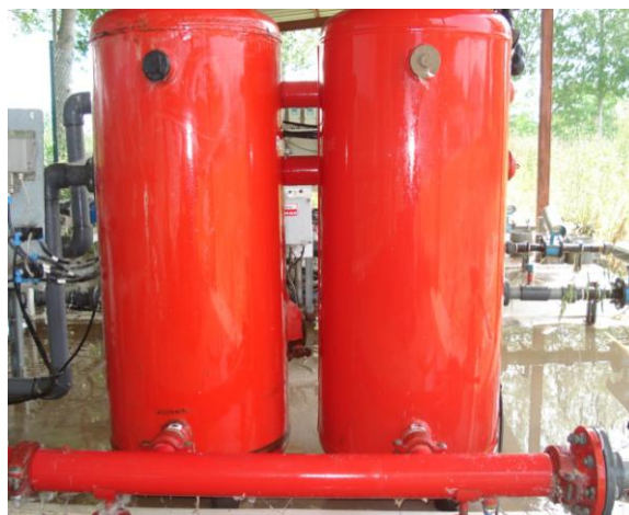
Fig. III-2. Filtration unit consisting of two sand filters in parallel.
