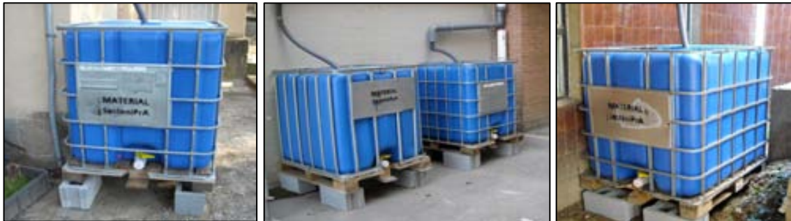
Figure 2.12. Rainwater tanks installed in the set of roofs in UAB campus (from left to right: rainwater tanks in CT, M, P and FG roofs).
