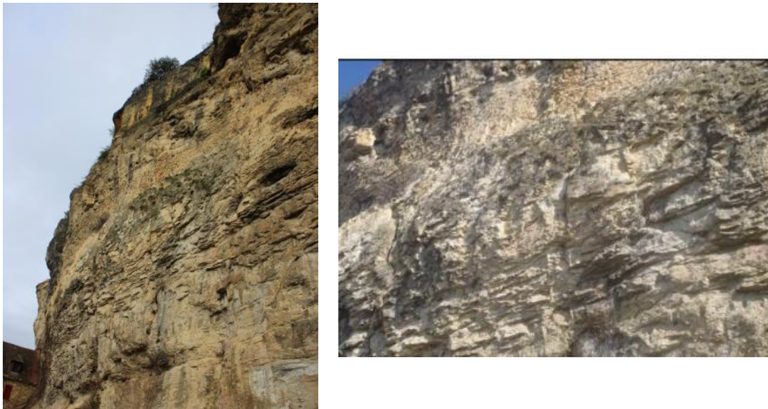
Figure 2-9 Flaking observed in the face of the cliff
