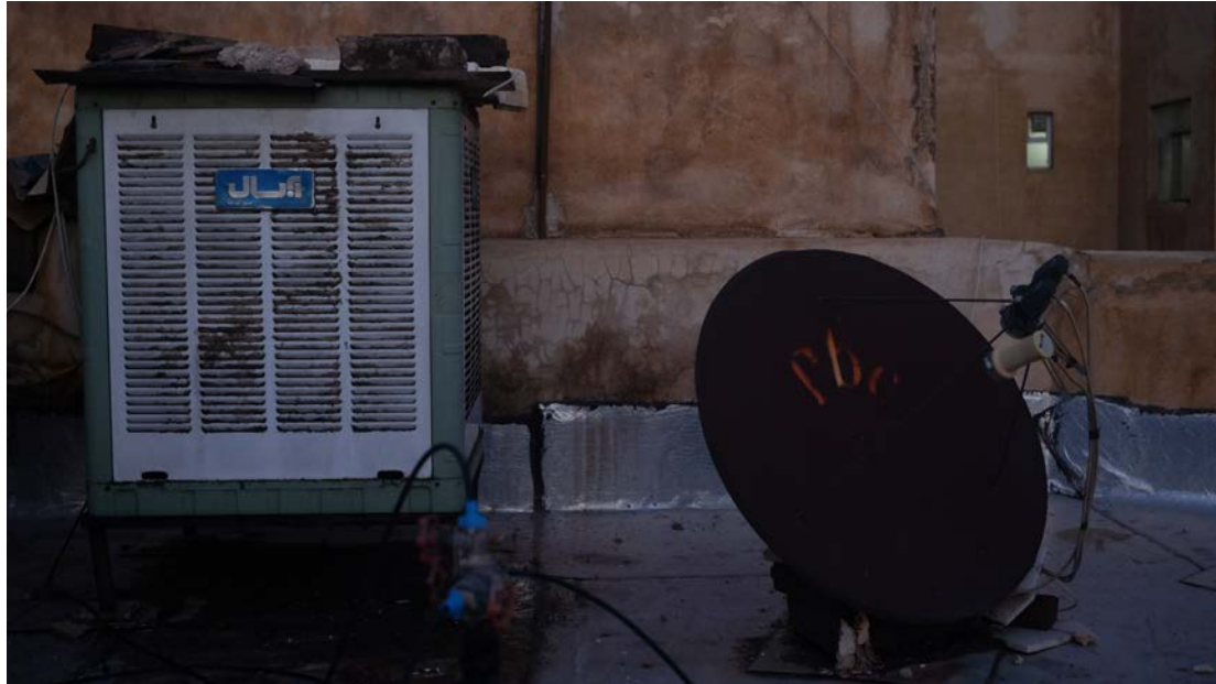
A cooler and an antenna on a roof in Tehran, October 2015
