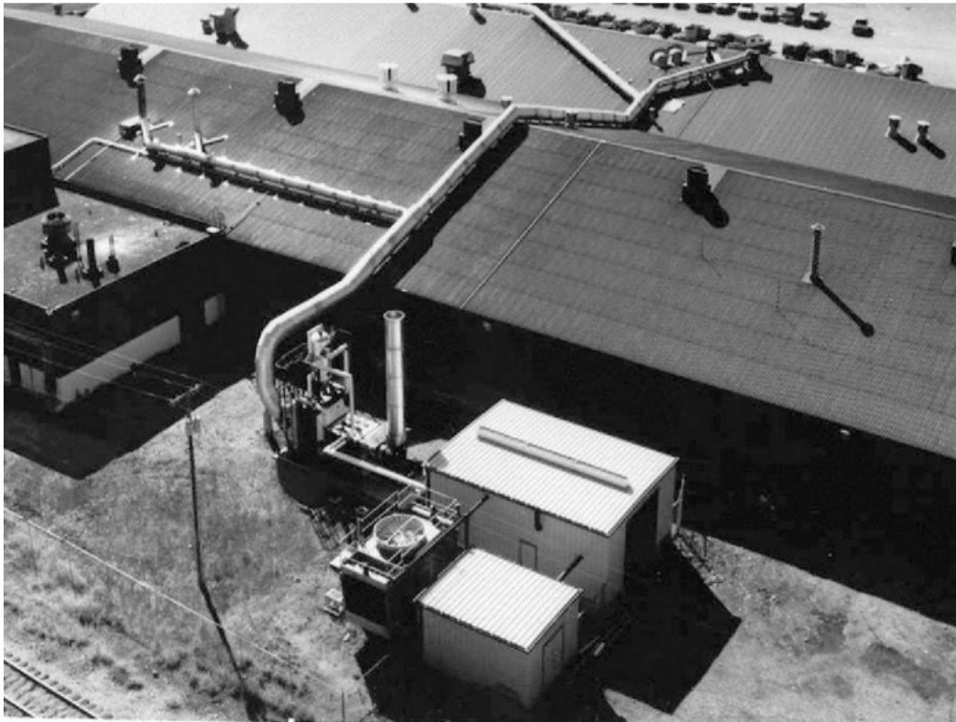
Fig. II.22. ORC plant of 500 kW. Heat source of hot gases collected with pipes from several ceramic kilns, Sundstrand 1983. (Source: Ref. [130])
