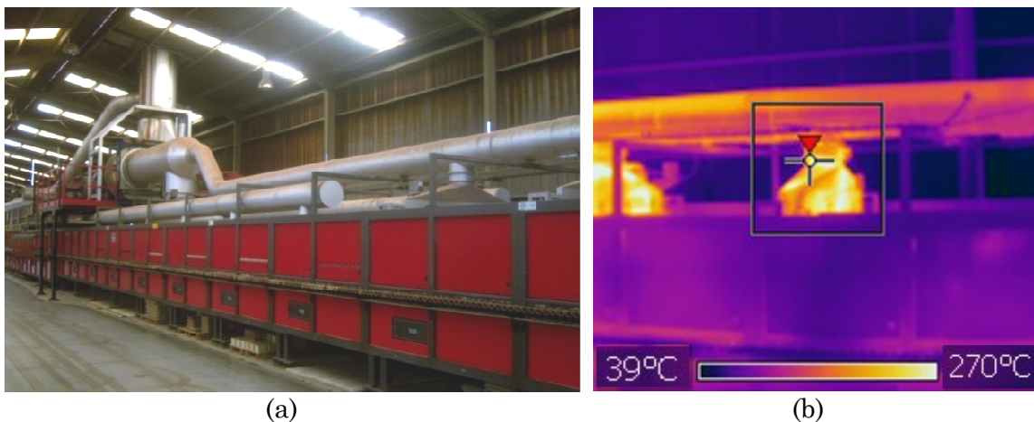
Fig. III.2. Intermediate cooling zone: (a) image of the original duct, (b) out of scale thermography of the duct.
