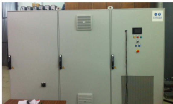
(a) Outer electrical cabinet view
