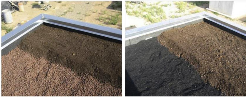
Figure 12. Substrate used in the extensive green roofs; left, view of the substrate over the pozzolana drainage layer, right, view of the substrate over the rubber crumbs drainage layer
