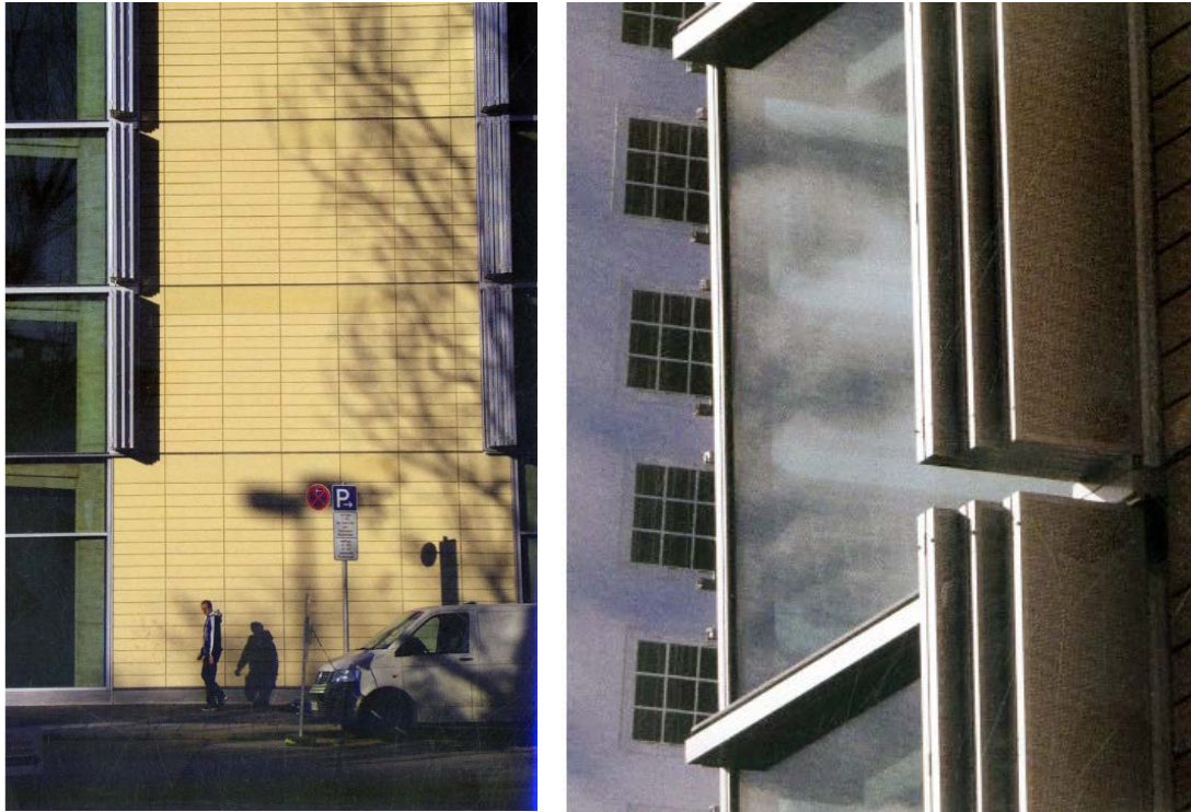
Figure 27: Oskar von Miller Forum, cladded walls with rear-ventilated, thermally insulated ceramic facade panels
