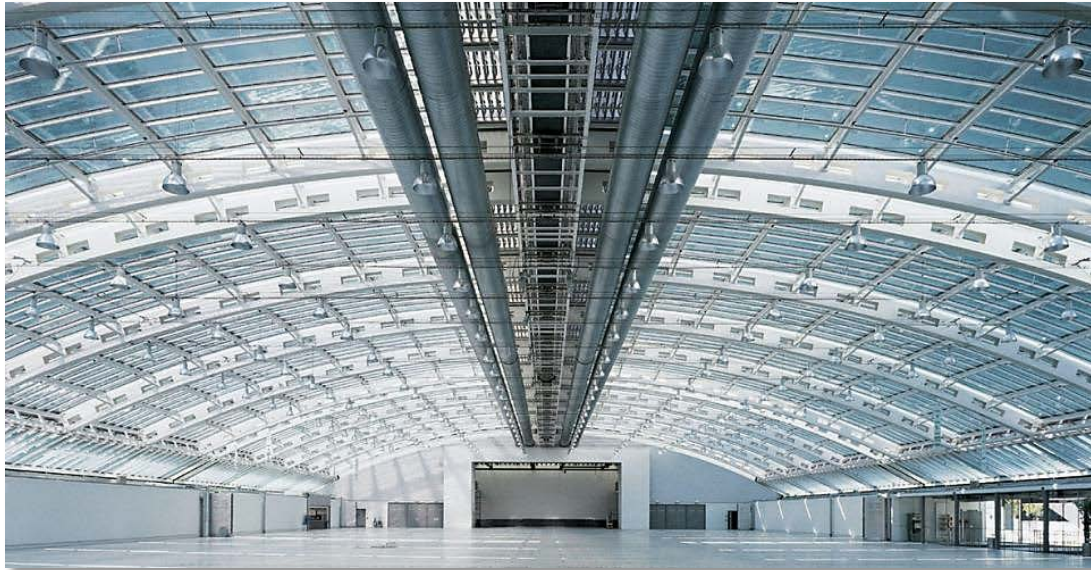
Figure 44: Exhibition hall in Linz, Distribution ducts installed under the center of the roof.
