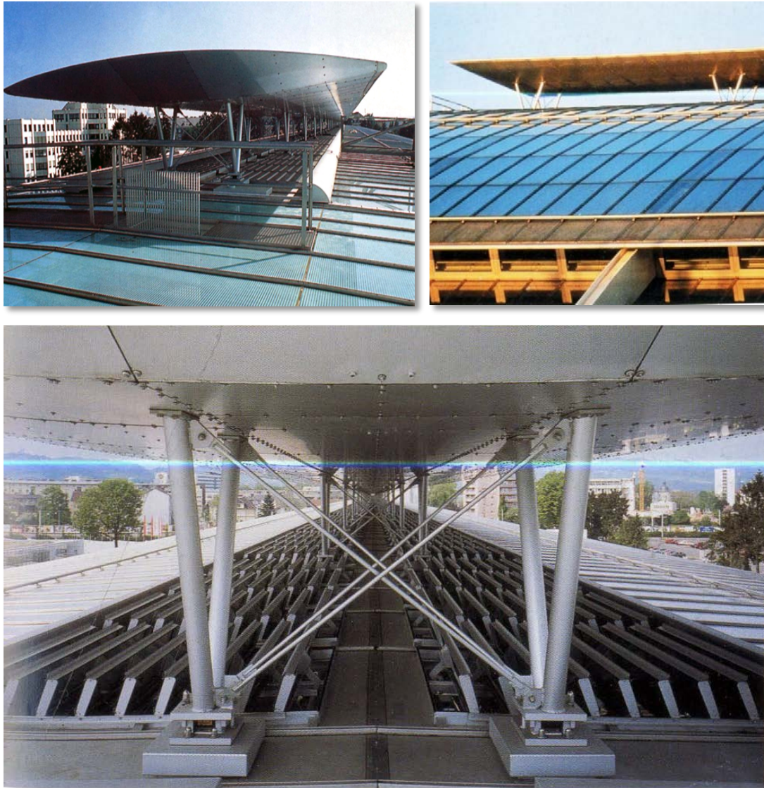
Figure 41: Exhibition hall in Linz, Ventilation elements with "Venturi" capping to assist natural ventilation
