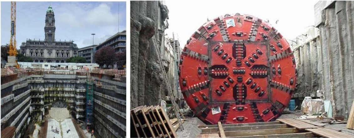
Figure 2.39 TBM breakthrough at Aliados station(left) and 8.7m diameter Herreknecht S-160 EPB Shield after assembly(Centis and Giacomini 2004).
