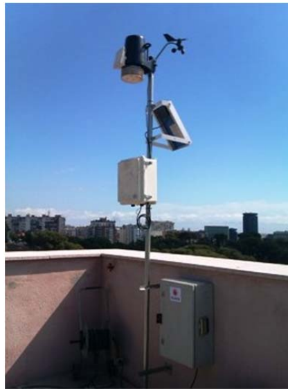
Figure 4.9 Weather station on K2M building.
