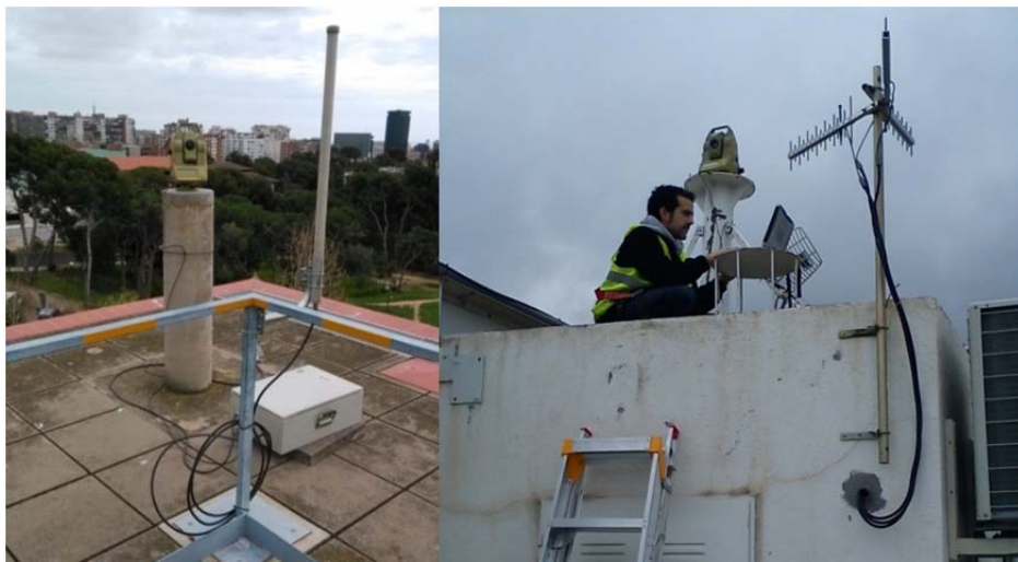
Figure 4.3 Example of RTS installed on A6-building (left) and N2-building (right) in UPC Nord Campus.
