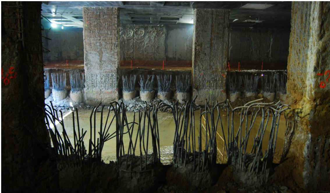
Figure 7.4. Picture of the interior of the station under construction. Construction stage corresponding to that shown in figure 7.3.c (Piles demolition between upper slab and parking level 1).
