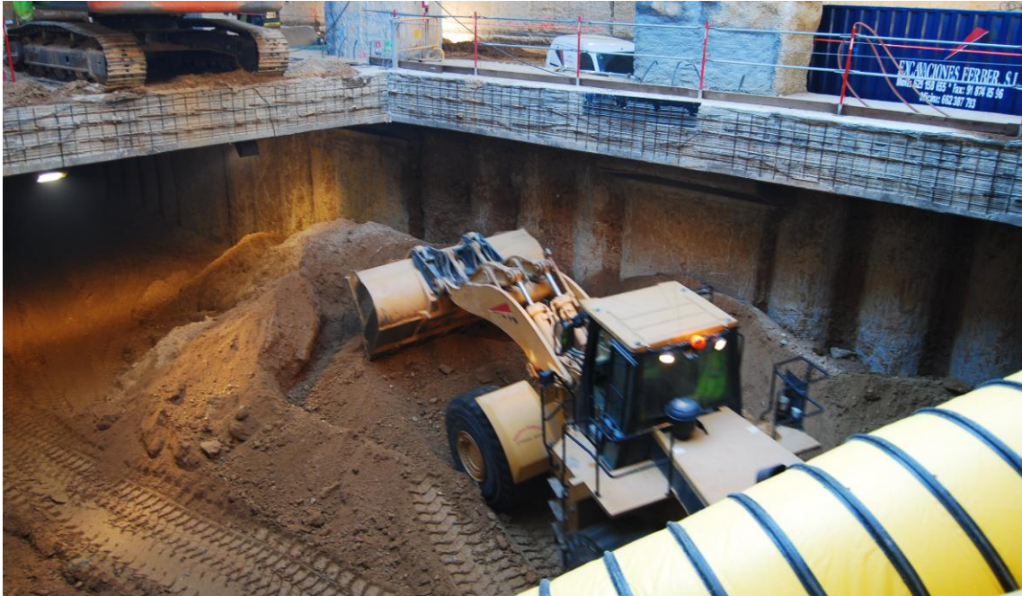
Figure 7.5. Picture of the interior of the station under construction. Construction stage corresponding to that shown in figure 7.3.e (7.285m of central excavation).
