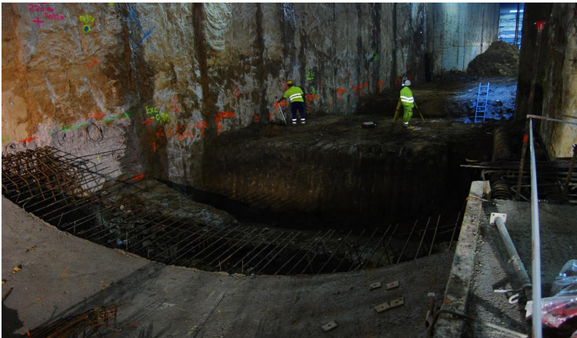
Figure 7.8. Picture of the interior of the station under construction. Construction stage corresponding to that shown in figure 7.3.o and 7.3.p (Lateral excavation to maximum excavation level and construction of the laterals inverted arches).
