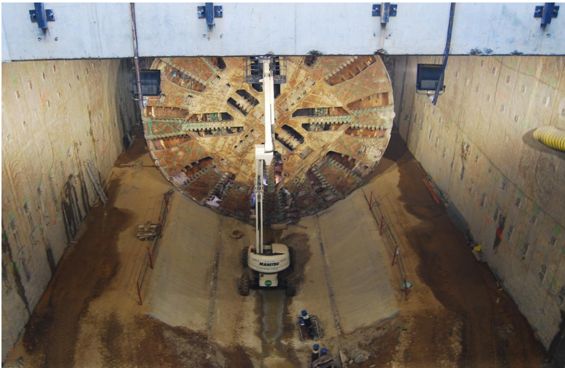
Figure 7.6. Picture of the interior of the station under construction. Construction stage corresponding to that shown in figure 7.3.h (Construction of the bus station slab and passing of the tunnel boring machine through the station).
