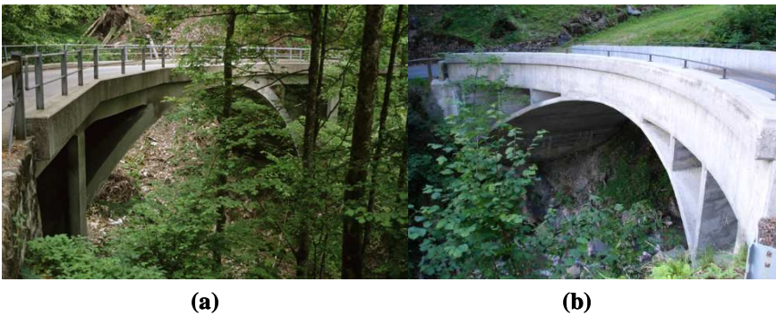
Figure 2-1: (a) Ziggenbach bridge ( Source: Yoshito Isono 1998. Reproduced by kind permission of Structurae (publisher) ); (b) Bohlbach Bridge; (c) Schwandwach Bridge ( Reproduced by kind permission of the author A. Ruiz-Teran )
