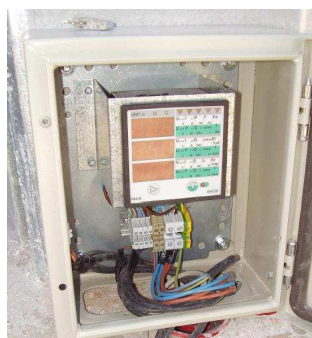
Figure 63. Electrical energy consumption measurement device.
