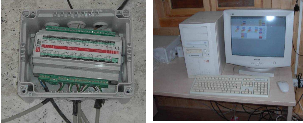
Figure 64. Data logger and computer installed in the cubicles.
