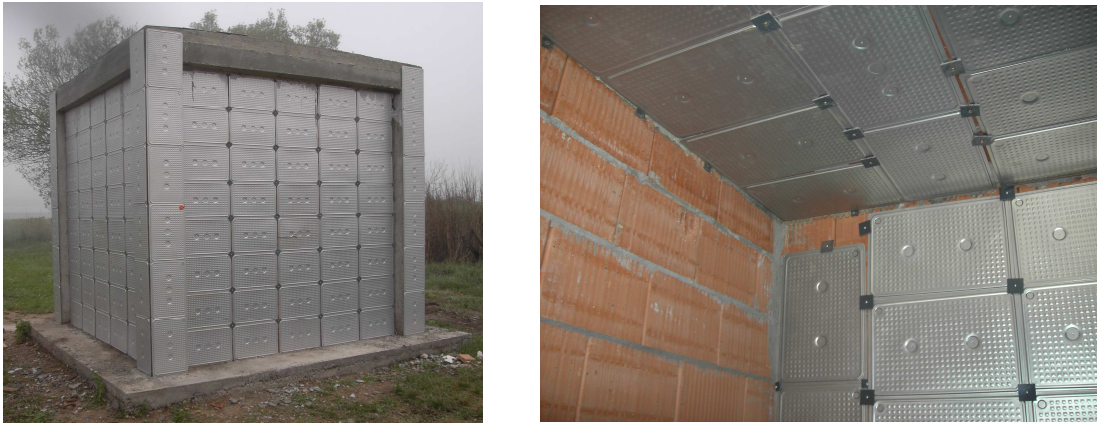
Figure 146. Brick cubicles with macro-encapsulated PCM: outer view (left); detail of inner view (right).
