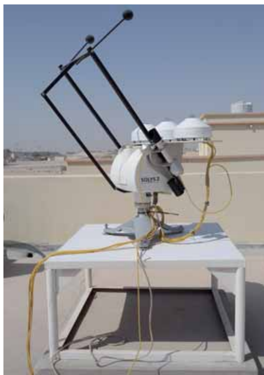
Figure 4.8: Solar radiation monitoring station as installed at the QEERI facility in Doha, Qatar.
