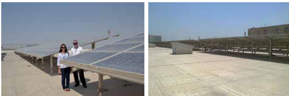
Figure 3.4: Photovoltaic panels on the roof top of the Qatar National Convention Centre.
